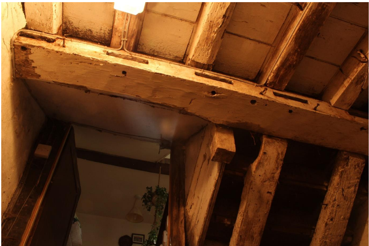
Figure 57 Reused timber incorporated into the underside of the farmhouse stair, looking south
