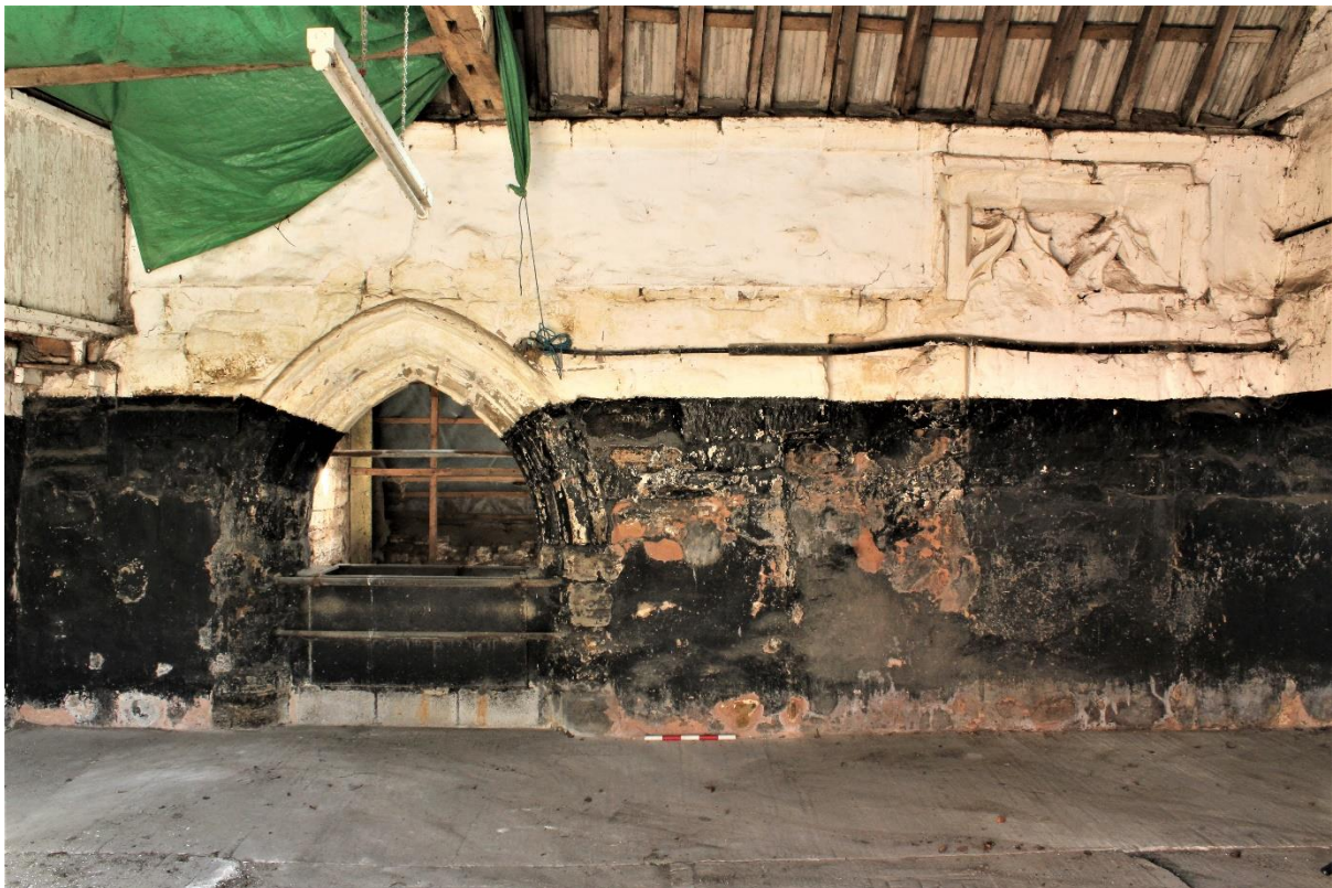
Figure 21 West elevation of the great hall, looking west, note the moulded doorway (left), blocked tracery window (right) and cornice (above)
