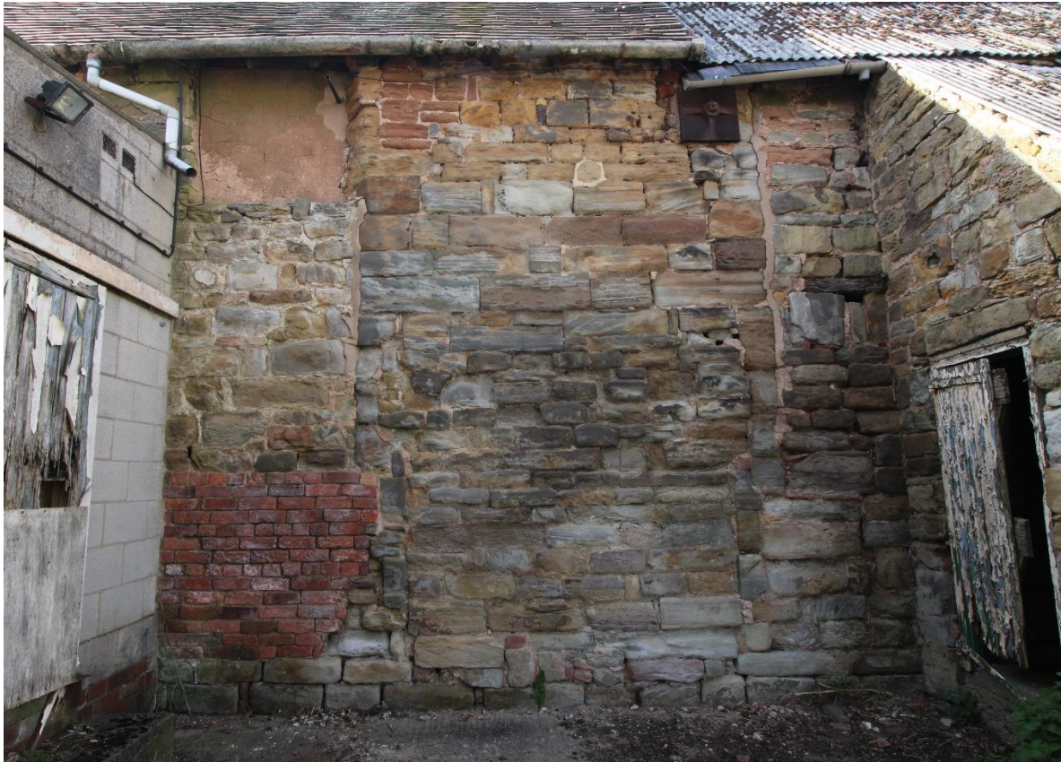
Figure 24 Detail of the east elevation of the mediaeval courtyard wall, looking west, note the straight joints of two blocked windows which flank the straight joints of a possible blocked fireplace
