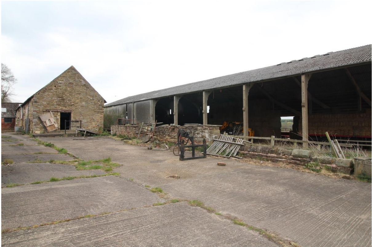
Figure 44 South elevation of Building 5 (left) and west elevation of Building 1 (right), looking north-east
