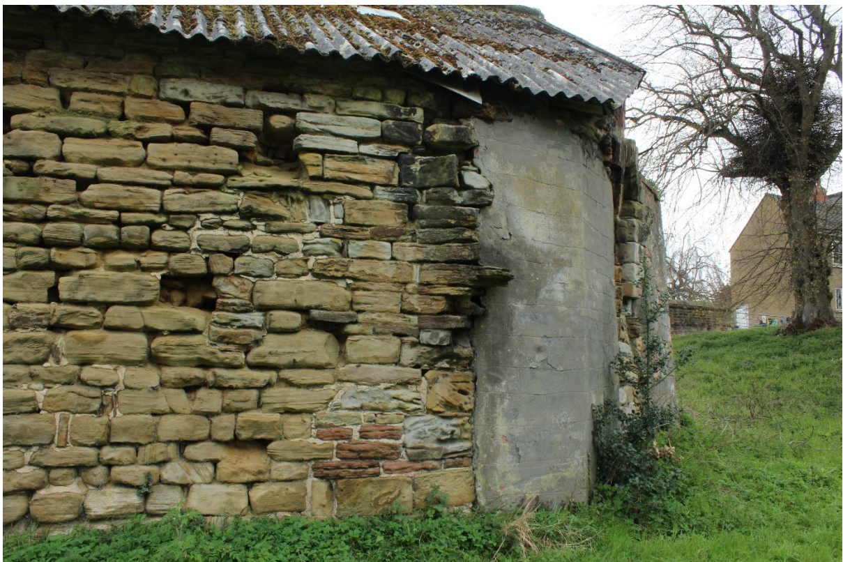
Figure 14 Projecting spur and blocked turret door at the west end of the north curtain wall, looking south-west
