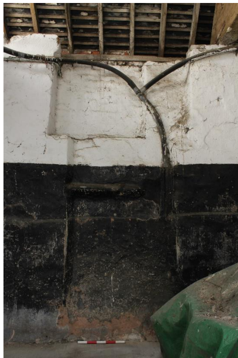
Figure 23 Blocked window in the west elevation of the great hall, looking east, note the truncated transom
