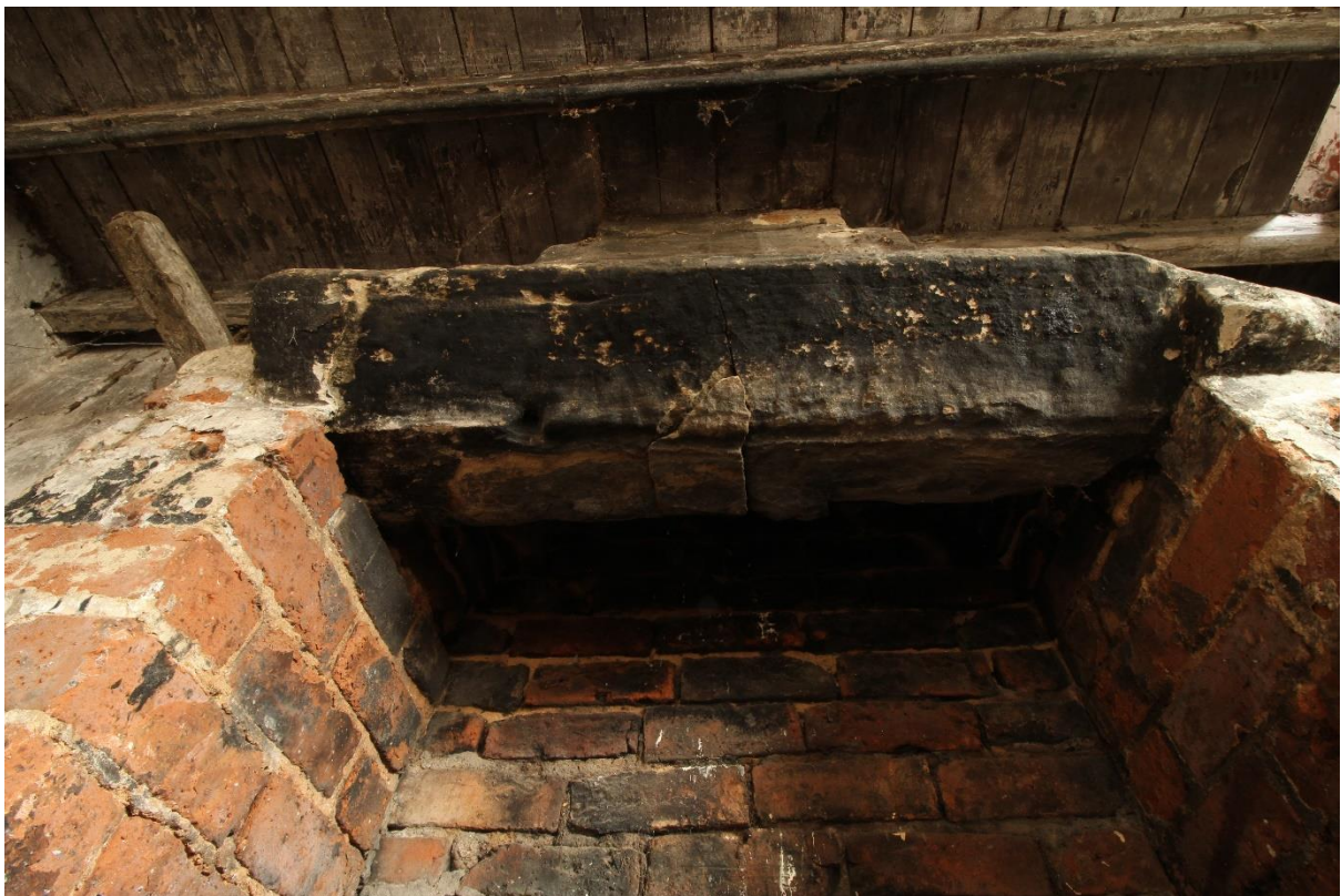
Figure 31 Window jamb reused as a chimneypiece in Building 9 (Ex Situ Feature Number 007), looking north
