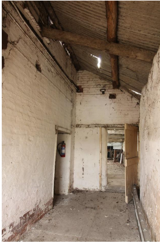
Figure 48 Through-passage between the eastern yard and Building 8 at the north end of Building 5, looking west
