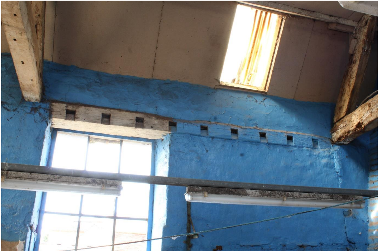
Figure 34 Floor beam reused as a window lintel in Building 5 (Ex Situ Feature Number 010), looking west
