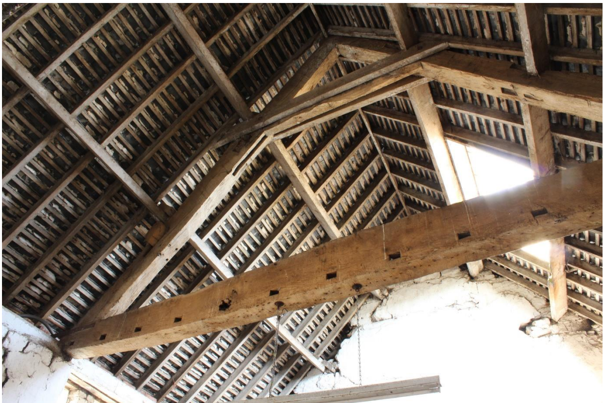
Figure 37 Reused timbers in Principal Truss 3, Building 5 (Ex Situ Feature Number 012), looking north
