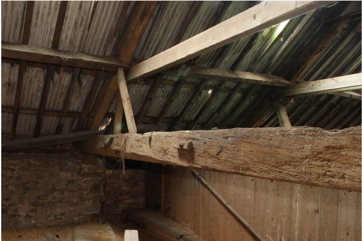
Figure 40 Reused timbers in Principal Truss 5, Building 5 (Ex Situ Feature Number 014), looking south-east
