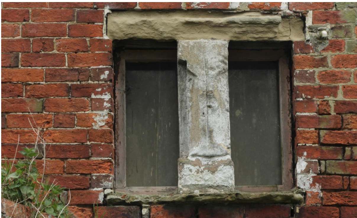
Figure 25 Window head reused as a mullion in Building 8 (Ex Situ Feature Number 001), looking east
