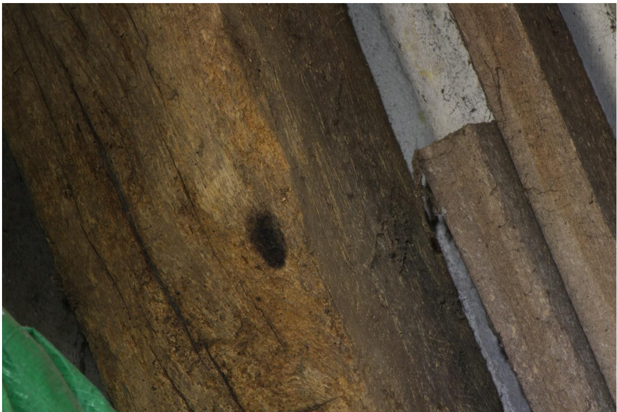
Figure 39 Possible apotropaic burn mark on the soffit of east rafter of Principal Truss 4, Building 5 (Ex Situ Feature Number 013), looking north-east
