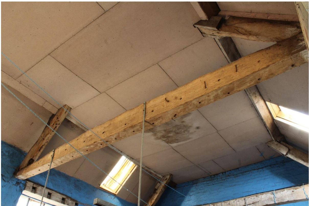
Figure 35 Reused timbers in Principal Truss 1, Building 5 (Ex Situ Feature Number 011), looking north-west
