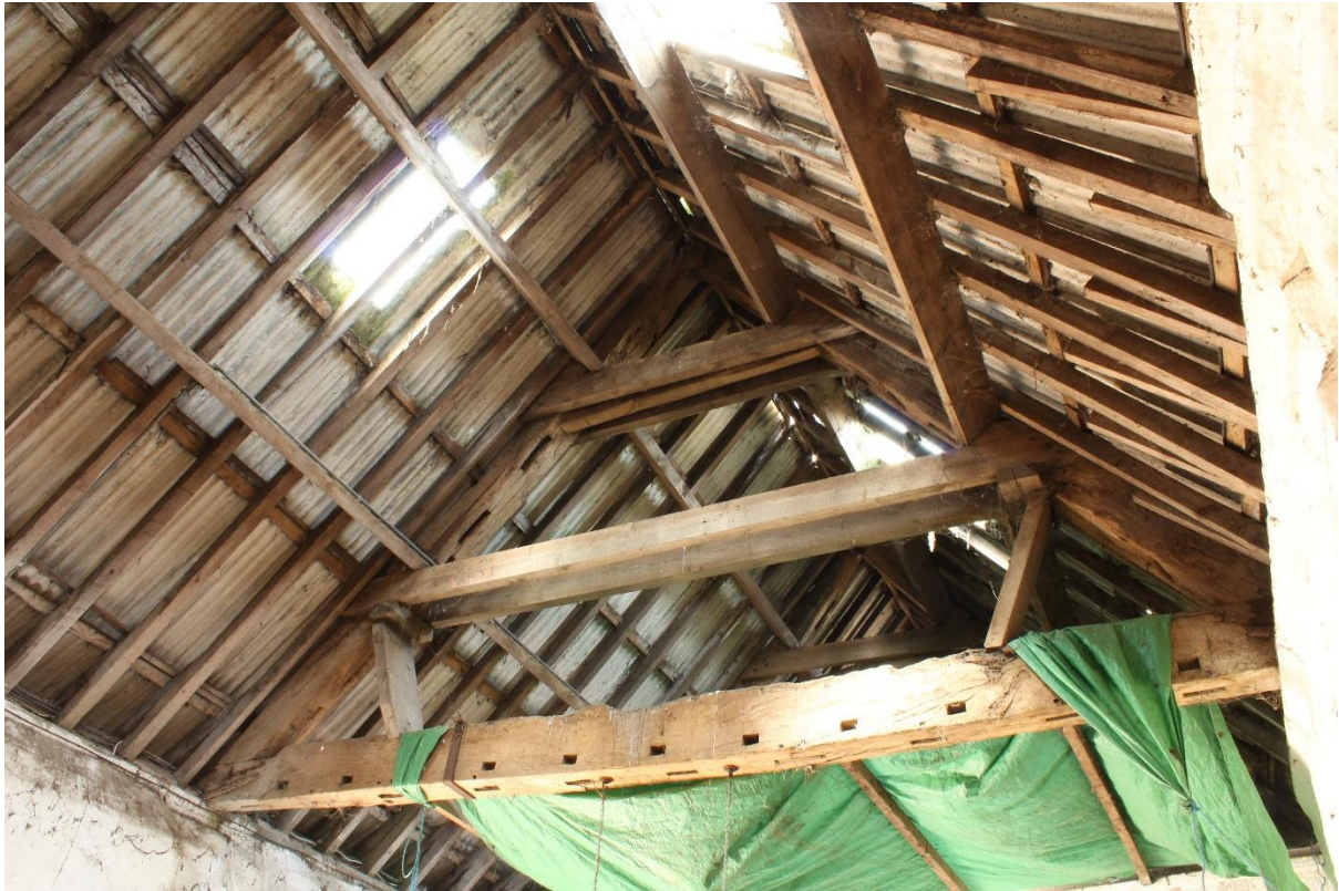
Figure 38 Reused timbers in Principal Truss 4, Building 5 (Ex Situ Feature Number 013), looking north
