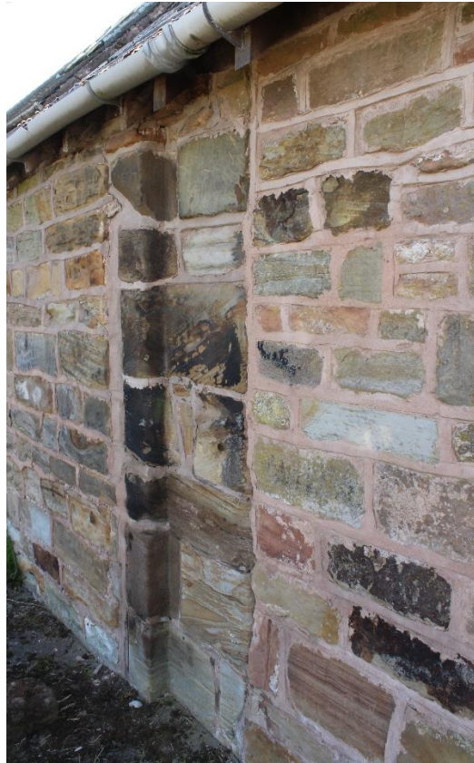
Figure 20 Door jamb of the east-west wall to the north of the moulded doorway, looking south-west
