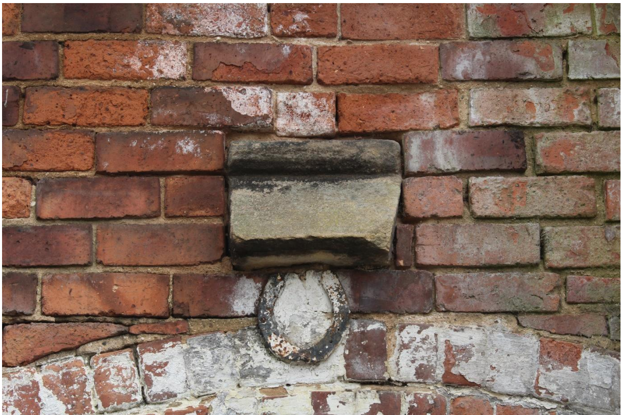
Figure 29 Moulded coping - possibly from a merlon - reused above the west farmyard entrance (Ex Situ Feature Number 005), looking east
