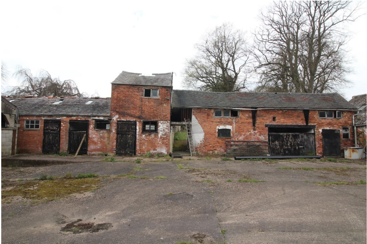
Figure 88 Exterior of the east elevations of Building 11 (left) and Building 9 (right), looking west
