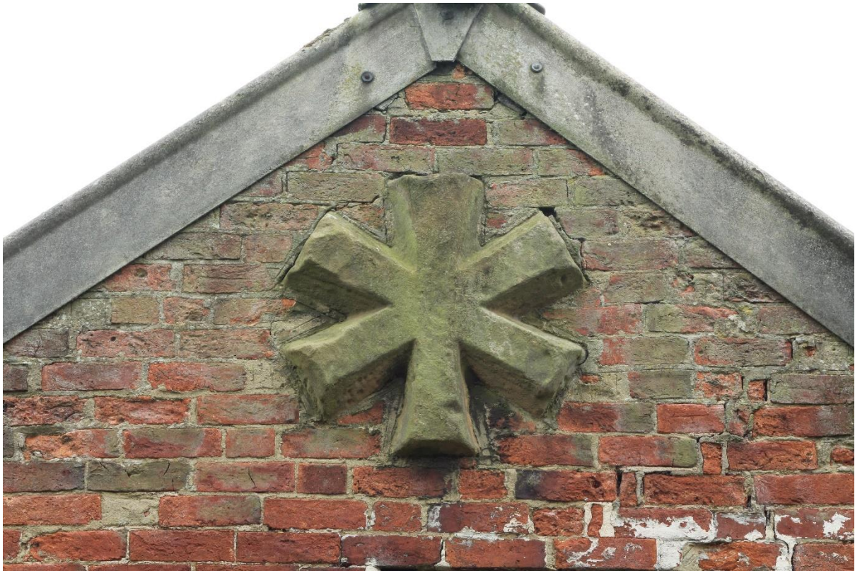
Figure 26 Crown of sexpartite vault reused in the gable of Building 8 (Ex Situ Feature Number 002), looking east
