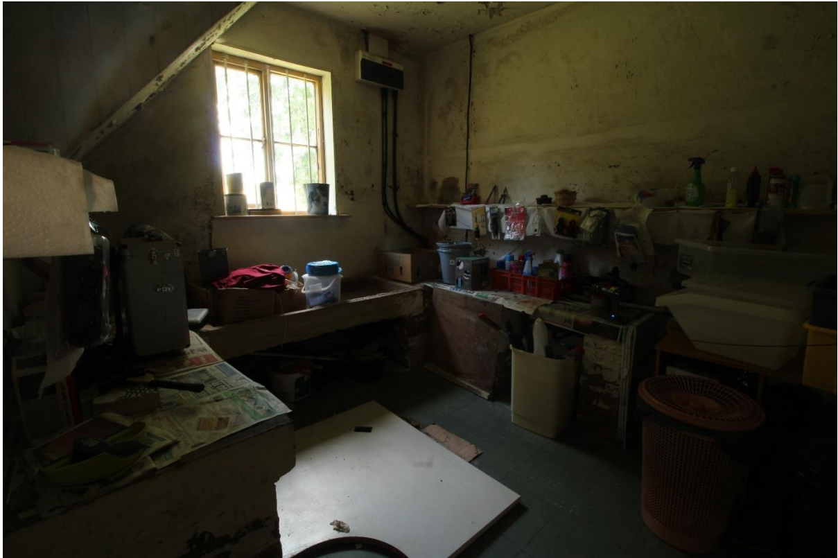
Figure 68 Possible former scullery or laundry in the farmhouse east extension, looking north-east
