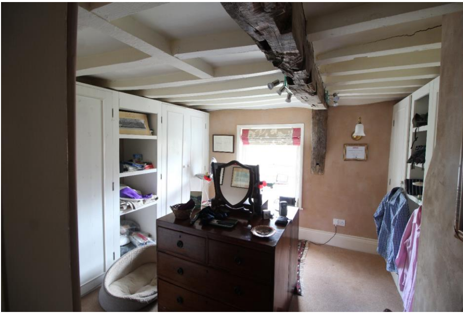
Figure 21 North-east bedroom at first floor of 12 Bell Lane. Looking east. Note the relict mortises in the spine beam.
