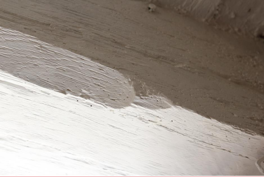
Figure 35 Chamfer stop of the western kitchen bridging beam at 6 Westfield Lane. Looking west.
