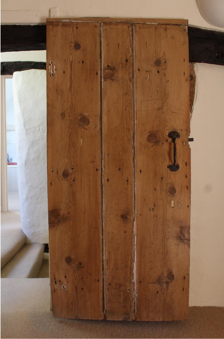
Figure 39 Outer face of the door between the stair and western bedroom at 6 Westfield Lane. Looking east.
