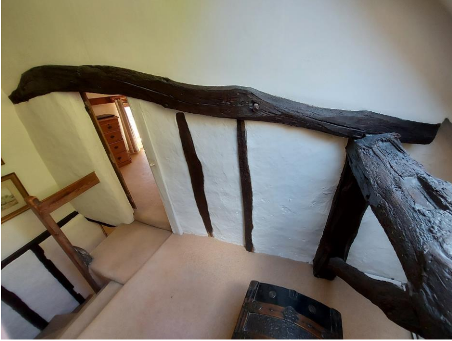
Figure 29 Transverse tie beam and wall studs (left) and longitudinal wall plate with brace and relict mortises for common rafters (right) at 6 Westfield Lane. Looking west.
