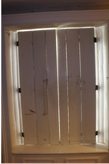
Figure 24 Window shuttering for the ground floor withdrawing room of 12 Bell Lane. Looking south.
