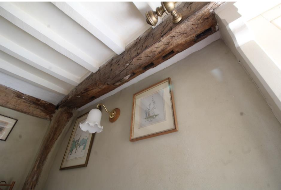
Figure 19 Soffit of south wall plate in south-east bedroom at first floor of 12 Bell Lane. Looking south-east. Note the relict mortises for wall studs.
