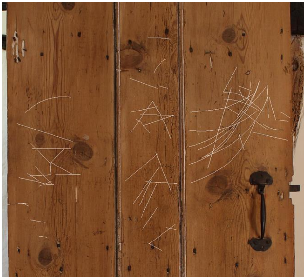
Figure 41 Scribed lines and arcs on the outer face of the door between the stair and western bedroom at 6 Westfield Lane. Looking east. Photograph has been interpreted with over-drawing.
