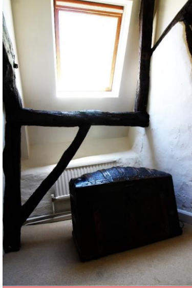
Figure 30 Post, bracing, wall plate and in situ common rafter at 6 Westfield Lane. Looking north.
