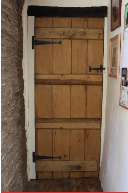
Figure 36 Door between the kitchen and living room at 6 Westfield Lane. Looking west.
